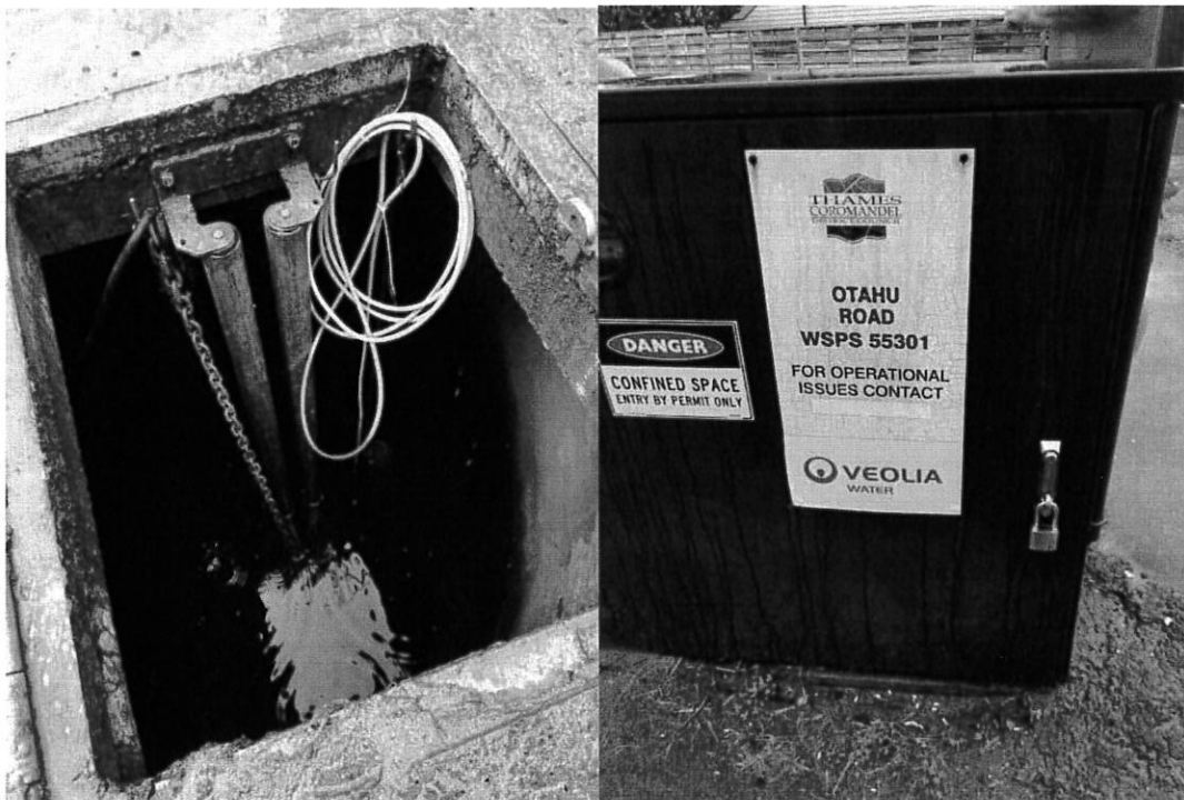
Figure 3-9 Otahu Road Pump Station
