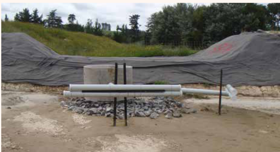
Sediment retention pond showing decant system.
